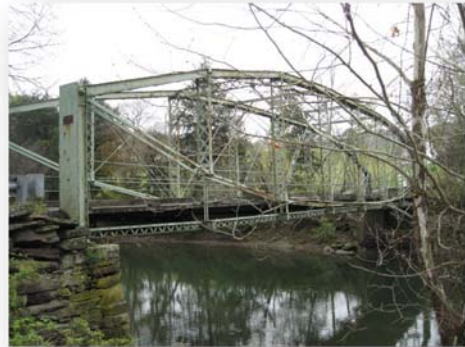
Lenticular Truss Before Rehabilitation
